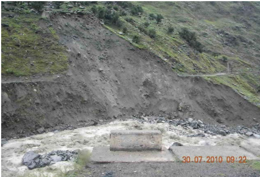
KKH Washed Away – Dubair
